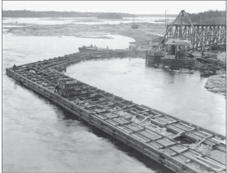
Rock-filled cribs were placed in the river to form a wall around the area to be drained dry. This area, called a cofferdam, is where the Seven Sisters Generating Station was eventually built.
