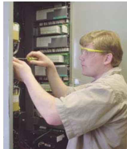
Dan Chevrier, energy systems specialist at Manitoba Hydro, checking a Pegasys power meter. The meter is one of 35 that gather the intelligence needed to manage loads efficiently throughout Inco’s complex.
