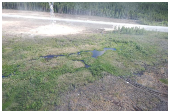
Photo 4: Evidence of minor damage due to vehicle traffic across a stream crossing.
