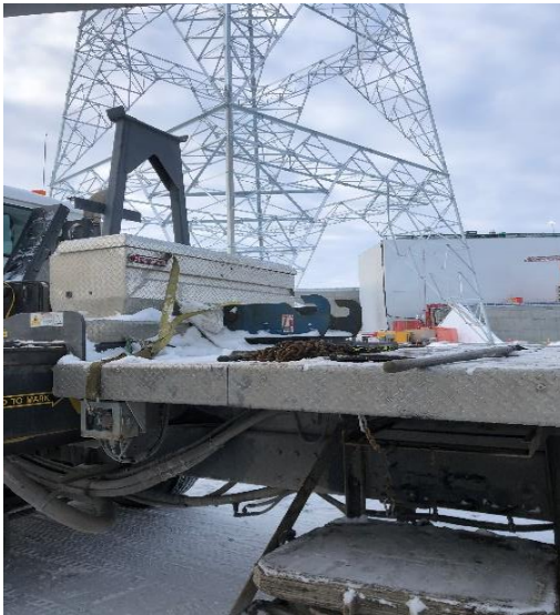
Photo 13: Environmental inspections were made of vehicles and equipment used on the construction site.
