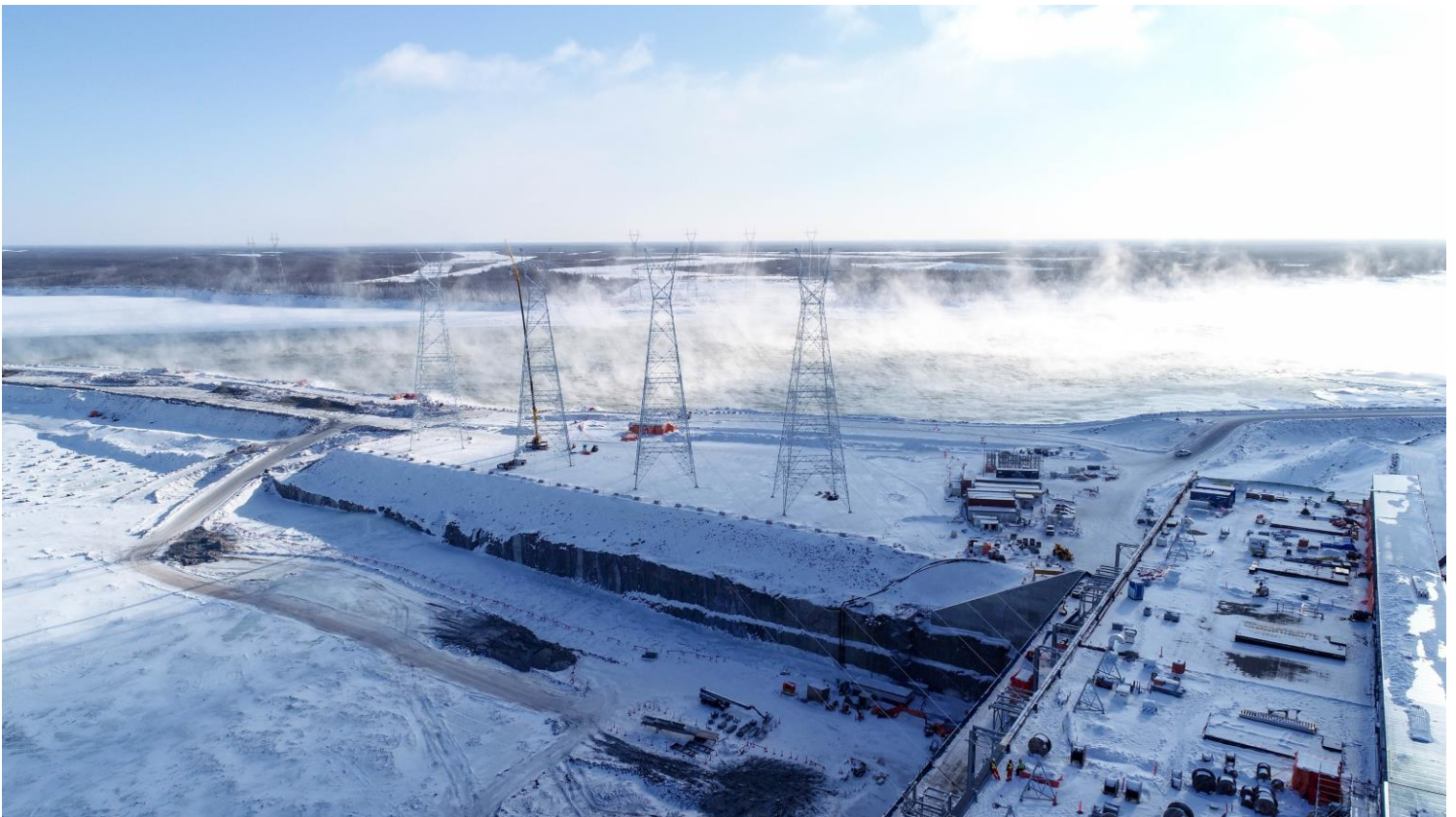
Photo 1: Keeyask Transmission Project is located south of Gillam, MB. Construction of the Project is now complete.
