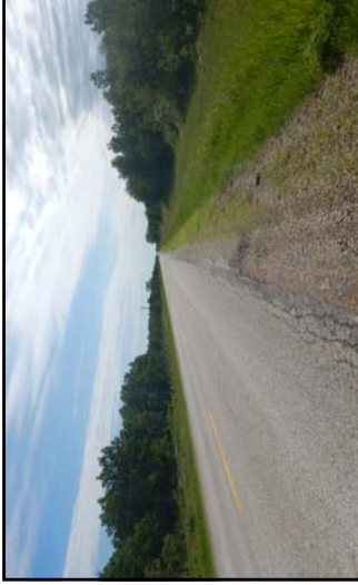
68RT- Facing East, ROW intersection with PR501. Culverts needed to cross steep ditch on both sides of the road to access ROW. Clearing required on both sides the ROW.
