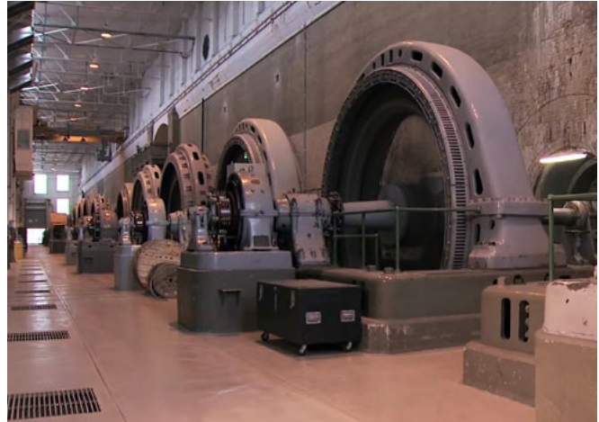
Based on current conditions, only three of the original 16 generating units are expected to operate beyond 2029.
