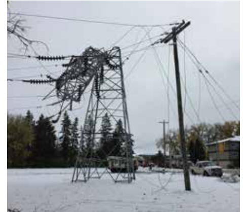
A steel tower in the Portage la Prairie area left crumpled by the storm.
