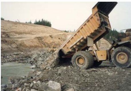
Figure 4.6-13 Typical Rock Fill being end dumped to close a cofferdam across a river.
