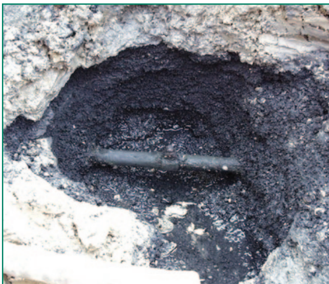
Above: Buried metal rod in coke bed from actual ground electrode
