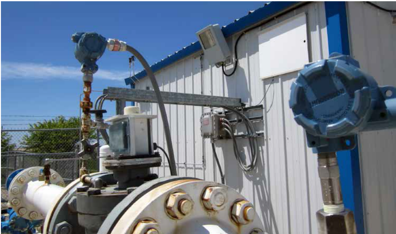
FIGURE 28 – PRESSURE MONITORING AT ST. NORBERT PRIMARY
