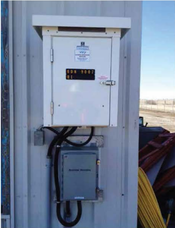
FIGURE 29 – RECTIFIER AND JUNCTION BOX
