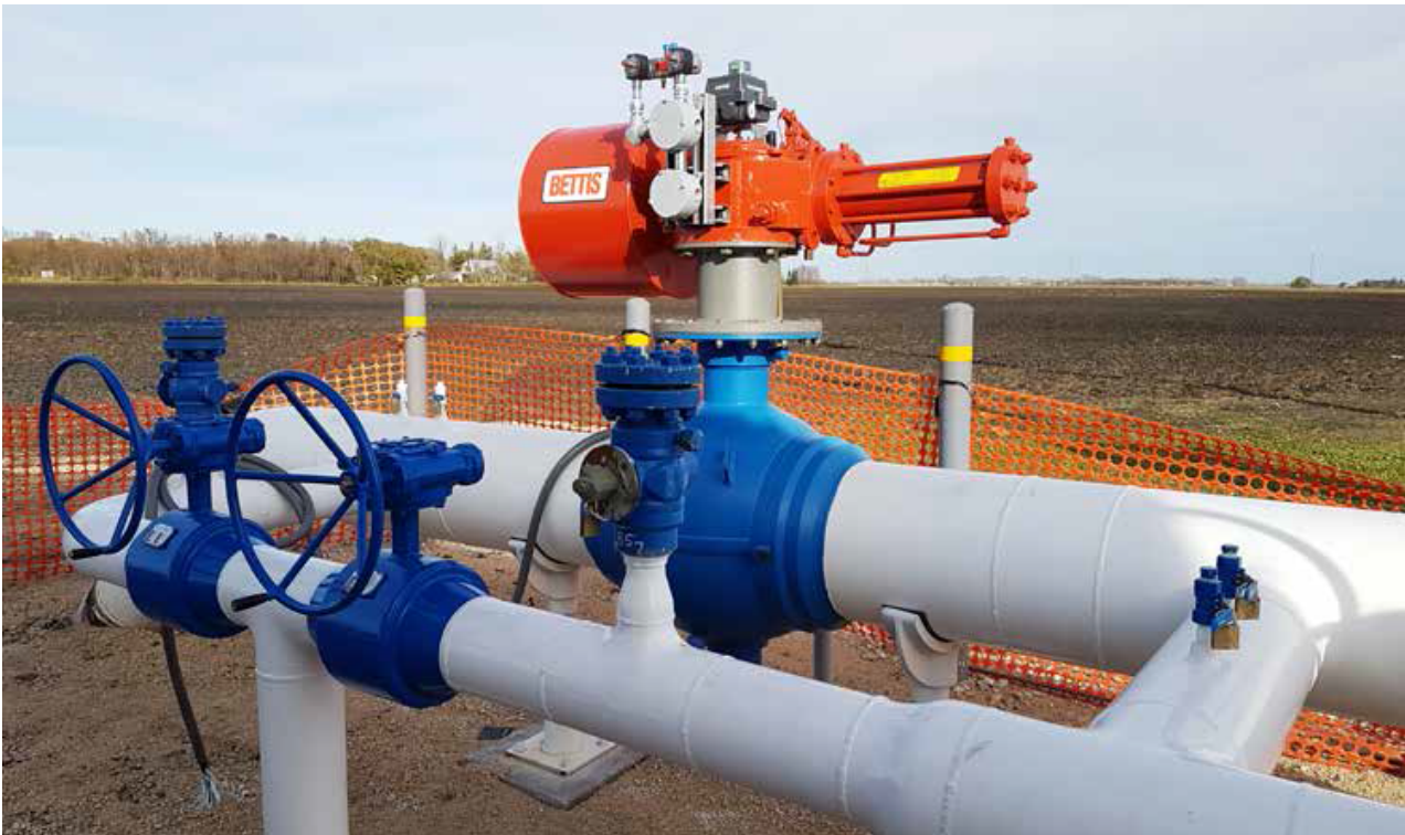
FIGURE 18 – T16-006 ACTUATED PIPELINE ISOLATION VALVE, IDC PIPELINE
