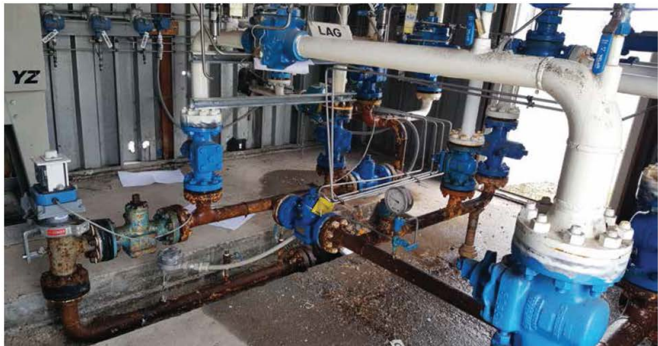
FIGURE 23 – EXISTING GS-018A LANDMARK PRIMARY GATE STATION, 2018 UPGRADE PLANNED
