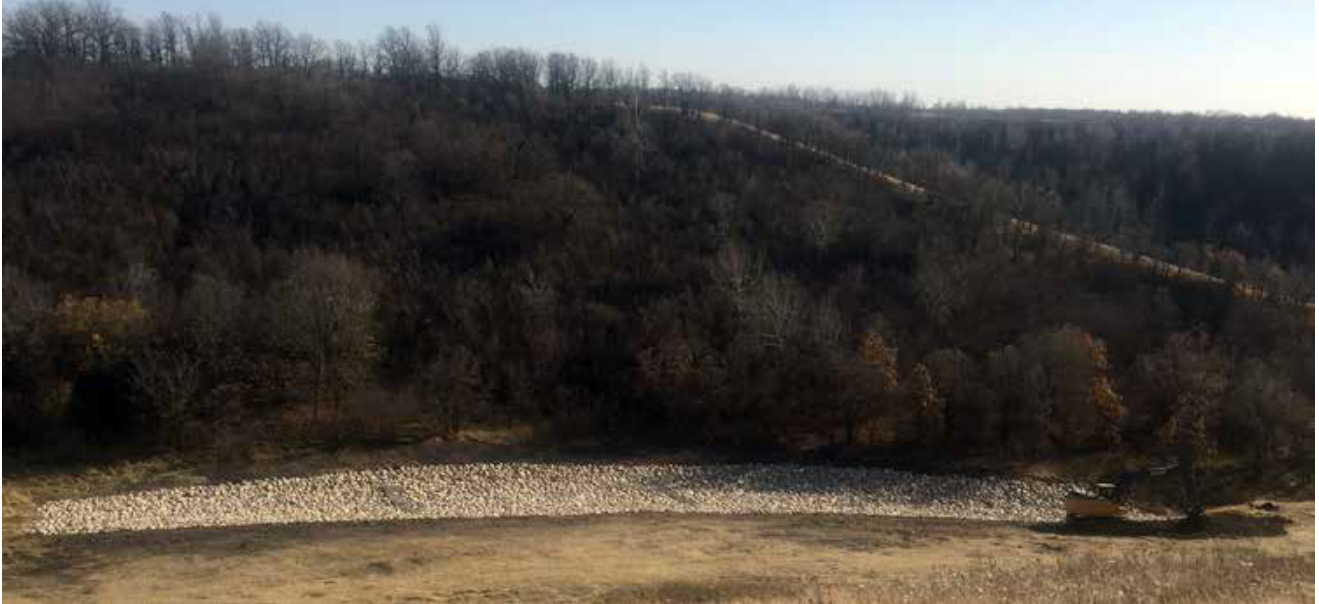
FIGURE 5 – INSUFFICIENT COVER REMEDIATION ALONG A STREAM TRIBUTARY FOR A PIPELINE CROSSING
