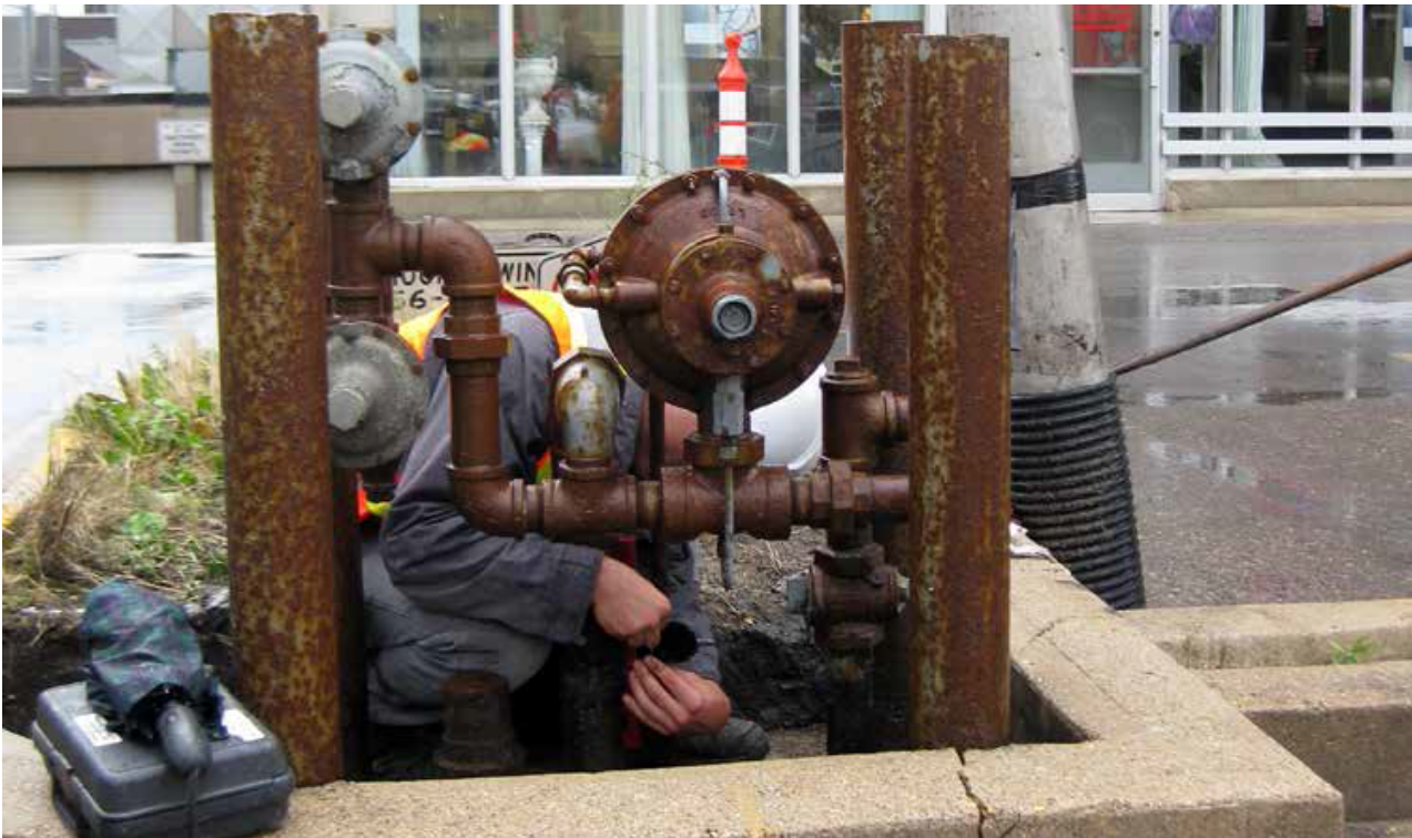
FIGURE 10 – EXAMPLE OF COMMERCIAL SERVICE REQUIRING REPLACEMENT DUE TO CORROSION
