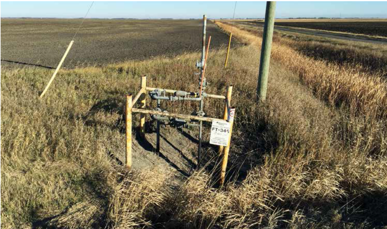
FIGURE 14 – FARM TAP REQUIRING UPGRADE
