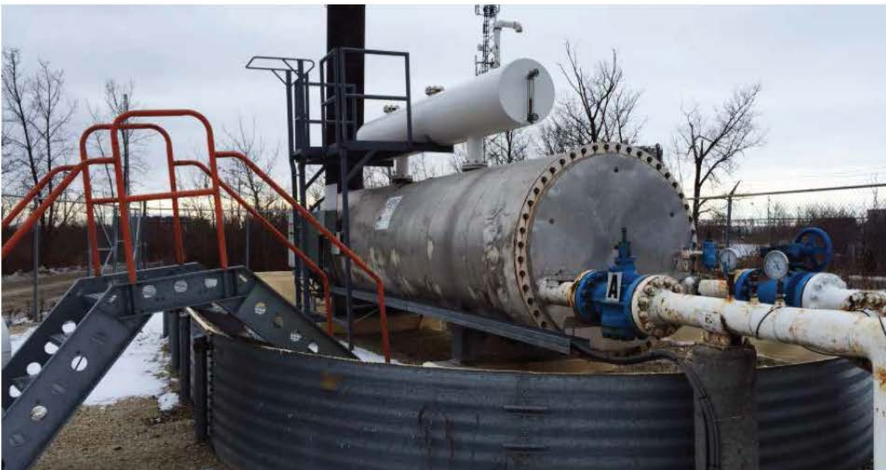
FIGURE 24 – GS-020 FORT WHYTE BATH HEATER WITH SECONDARY CONTAINMENT
