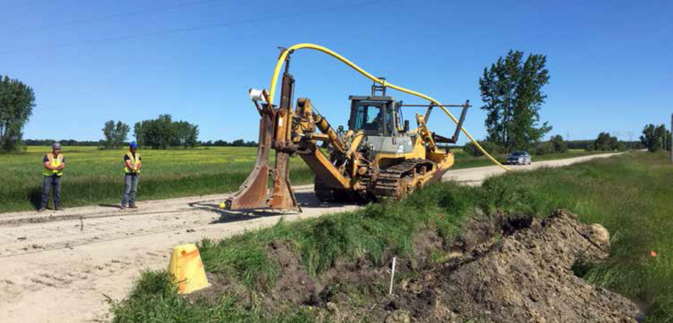
FIGURE 3 – PLOUGH PREPPED FOR INSTALLATION OF 114.3MM (4") POLYETHYLENE (PE) FOR A RURAL FARM SITE
