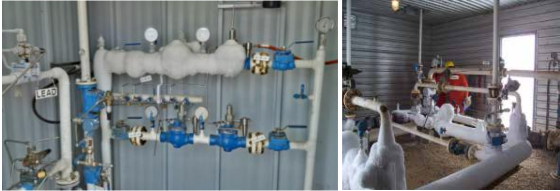
Figure 14: External icing on station piping due to the Joule-Thompson effect
