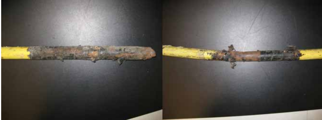
Figure 8: Corrosion leaks on service lines below polyethylene tape joint coating
