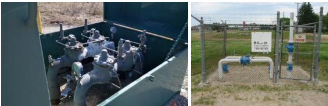
Figure 3 Regulator stations: box style (left) and inside fence style (right)
