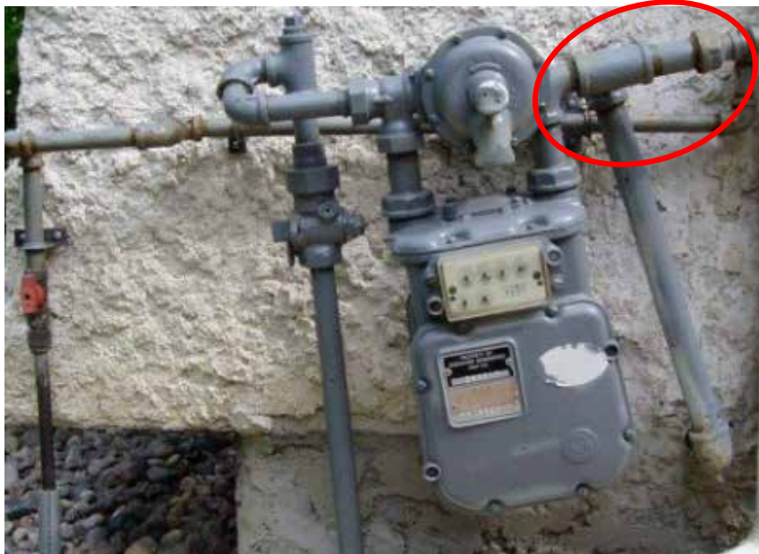
Figure 16: Auxiliary piping impeding swing joint movement
