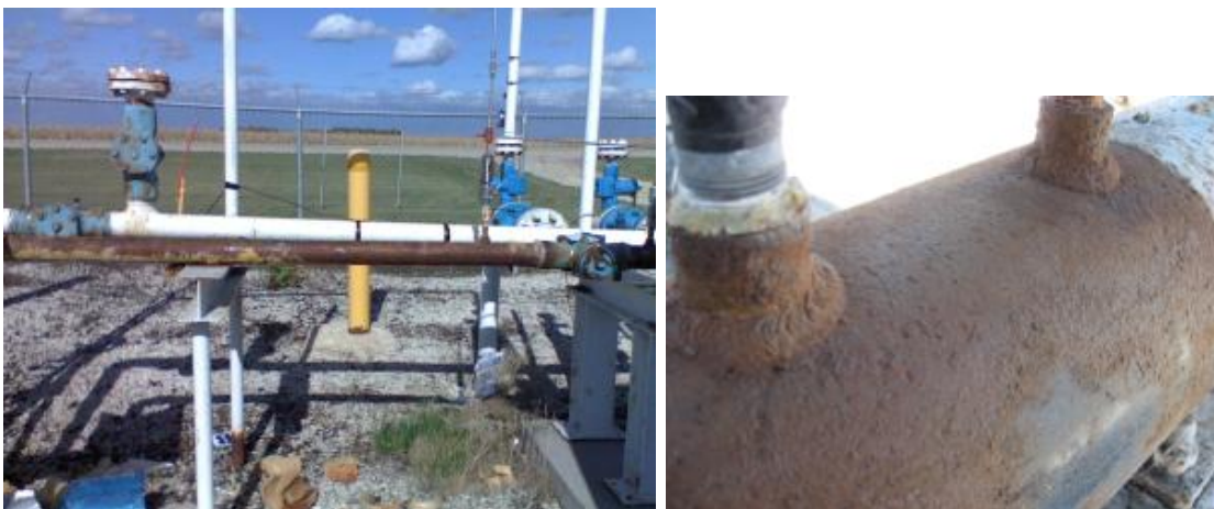
Figure 11: Corrosion under insulation at Ste. Agathe (GS-180) and Fort Whyte (GS-020)
