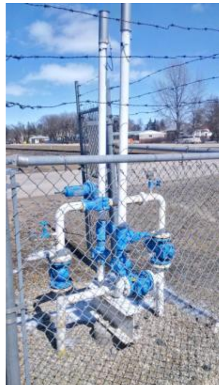
Figure 15: 630 Regulator Station in Gimli with Obsolete 630 Fisher Regulator
