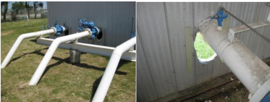
Figure 13: Heaving of piping and pipe supports causing damage to station building and stressing of pipe at Transcona Gate (GS-003)
