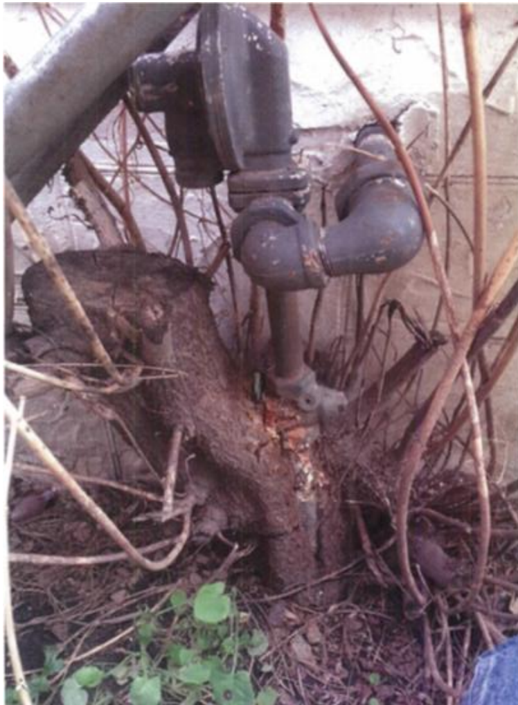
Figure 7: Riser in tree – accessibility issue with severe corrosion on inside meter set
