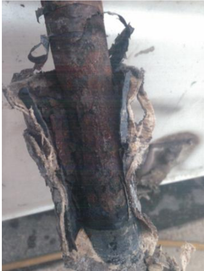
Figure 4: Above grade unsleeved riser with pipe corrosion under coating
