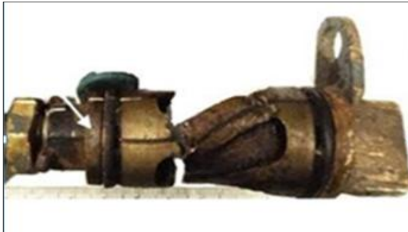
Figure 9: Damaged lub-o-seal valve
