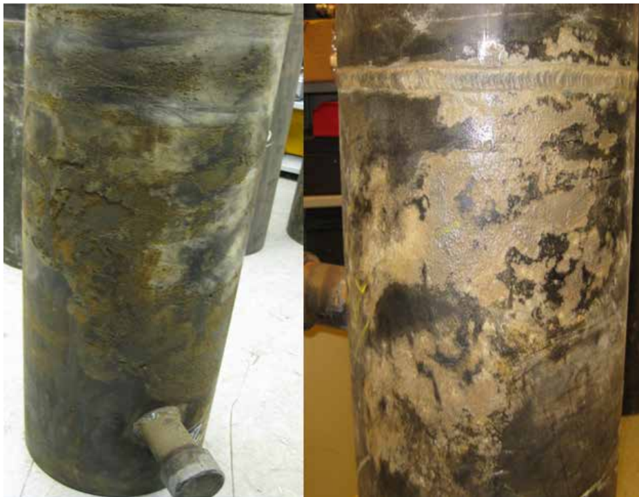
Figure 9: Cylinder of severely corroded pipe from below polyethylene tape joint coating
