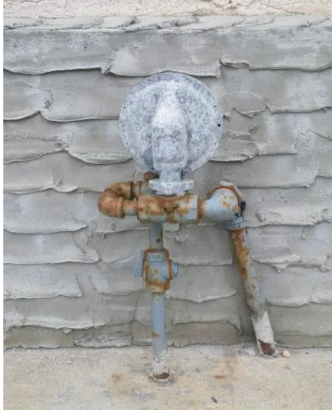
Figure 6: Corroded riser in concrete with below grade entry and delaminated coating
