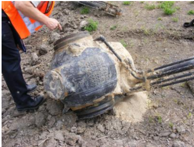
Figure 12: Vintage valve removed from service due to seizing.
