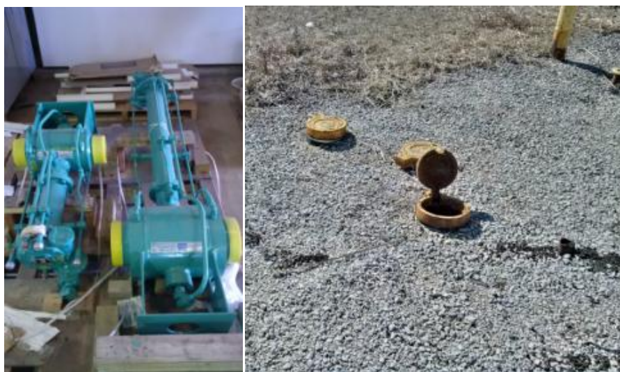
Figure 6: Below Grade Valves: Prior to installation (left) and installed with valve box cover visible (right)
