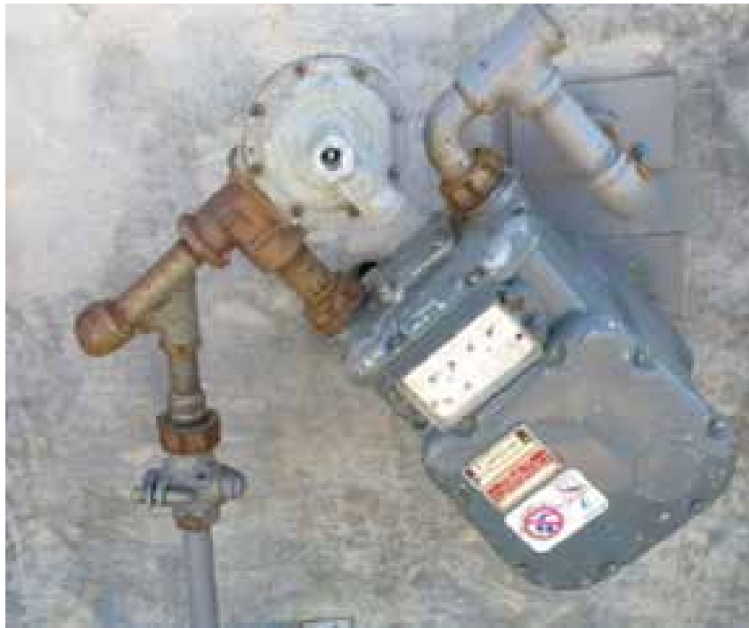
Figure 15: Residential service with inadequate swing joints causing strain on piping
