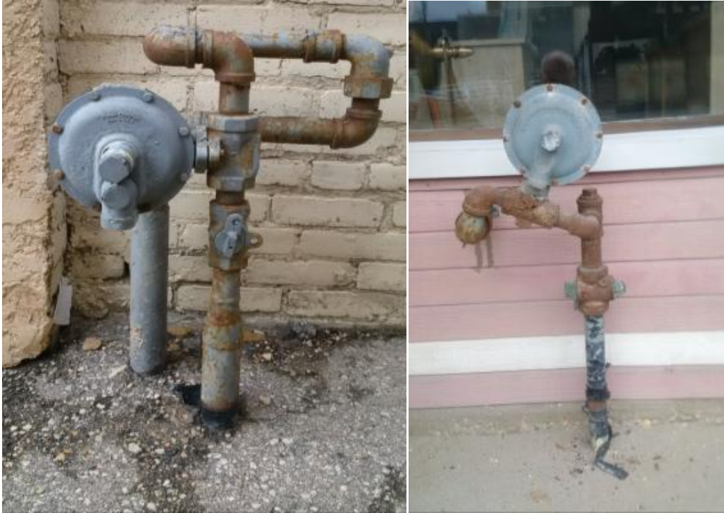
Figure 5: Below grade entry riser in concrete facing a high traffic area (left) and riser in concrete with degraded wrapping, corrosion and strain facing high-traffic area
