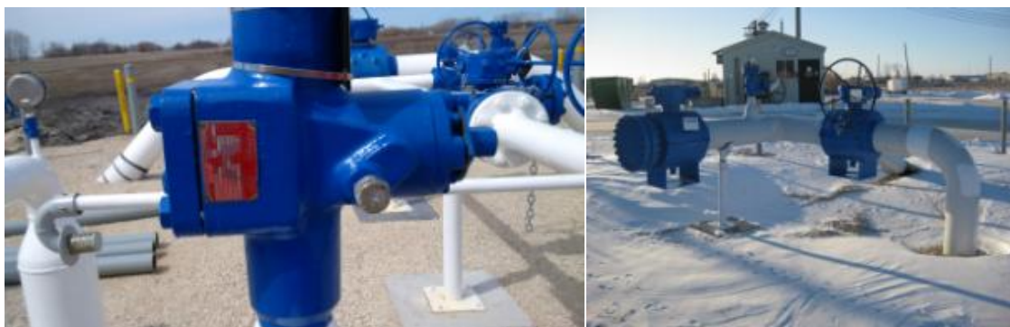
Figure 5: Above grade pipeline valves: Plug valve (left) and ball valve (right)
