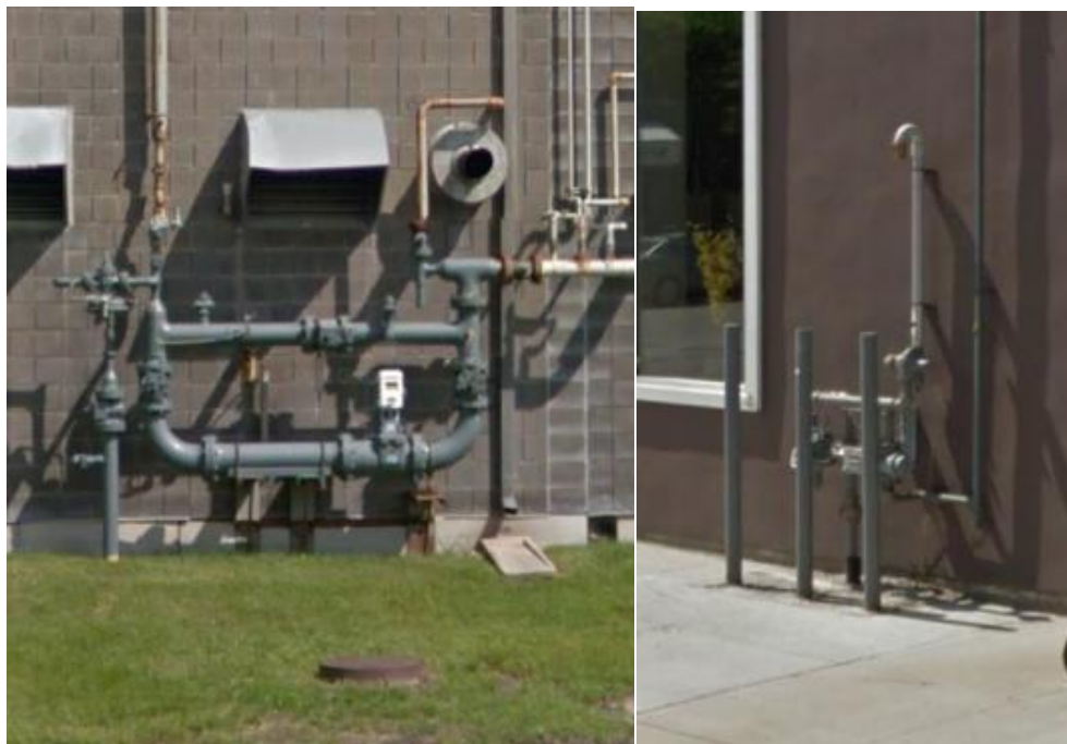
Figure 2: Example of large industrial service (left) and large commercial service (right)
