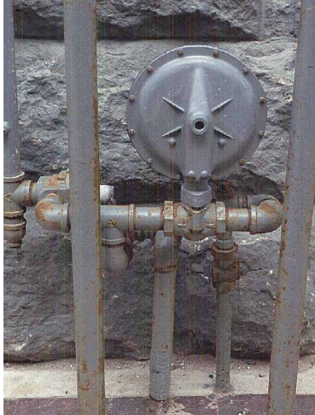
Figure 17: Commercial Regulator with Inside Meter Riser installation below grade entry
