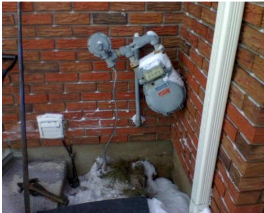
Figure 8: Residential service with “S” tube riser.
