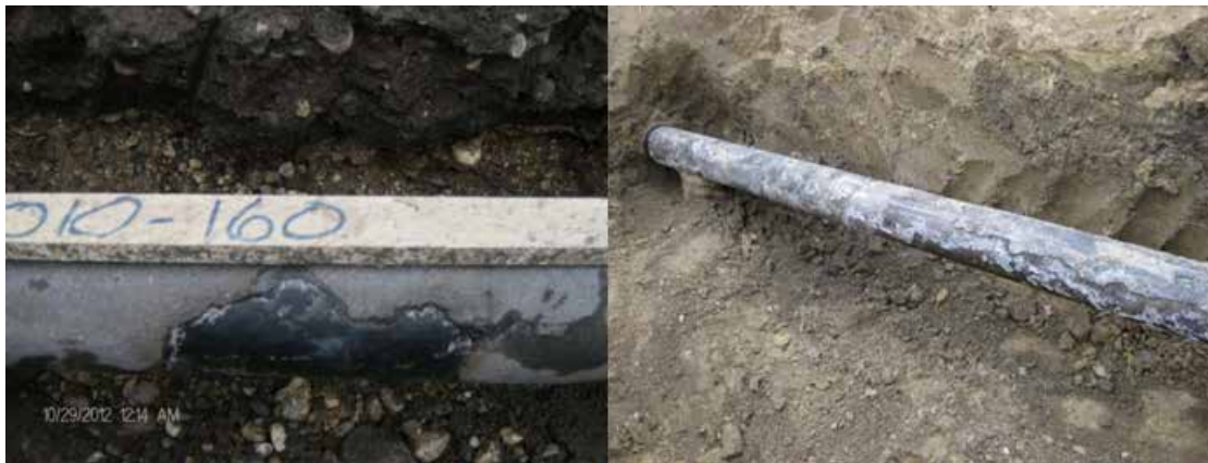
Figure 7: Deteriorated coal tar enamel coating on Shilo (left) and Dominion City (right) transmission pipelines.
