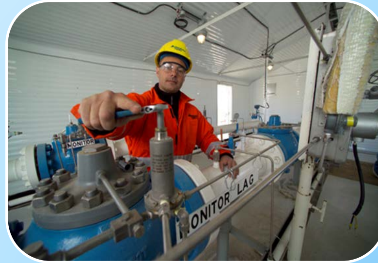
Energy Supply, Planning and Support
