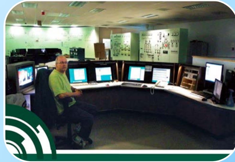
Natural Gas System Monitoring
