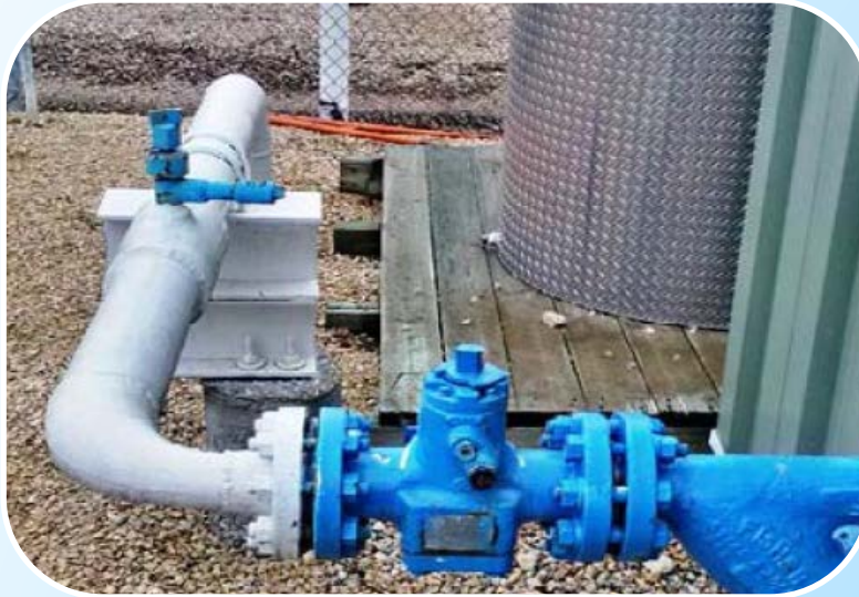
Natural Gas Pipeline Cathodic Protection
